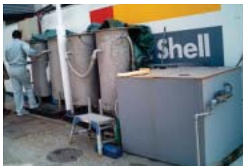
Bioreactor in place at a service station.
