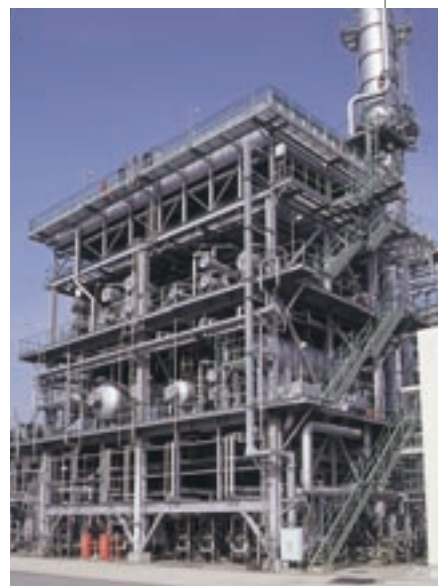
Benzene extraction facilities at Group refineries support Showa Shell's production of low-benzene gasoline.
