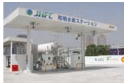
The Ariake Hydrogen Station
