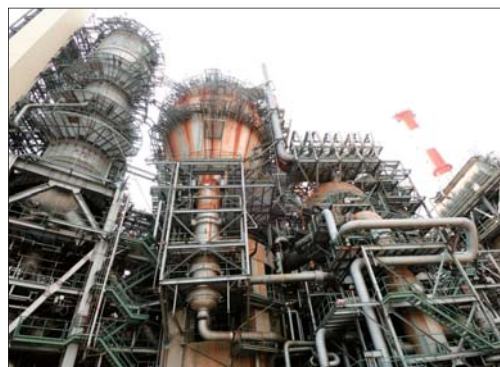
The Yokkaichi Refinery's residue fluid catalytic cracker (RFCC) produces high value-added products from heavy oil.
